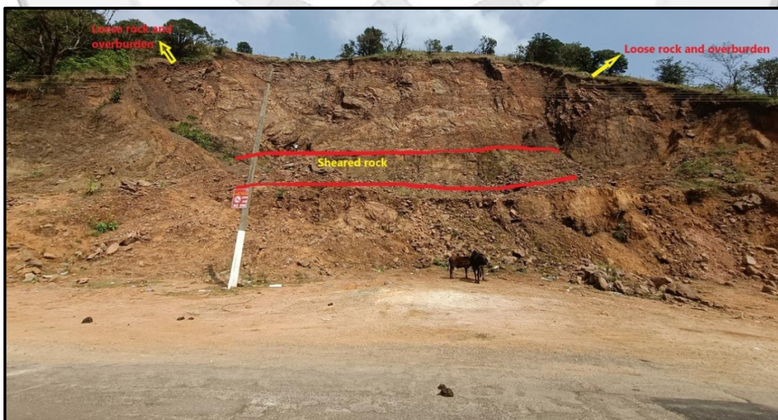
Fig. 4.9: Latest photograph of Talakaveri landslide
