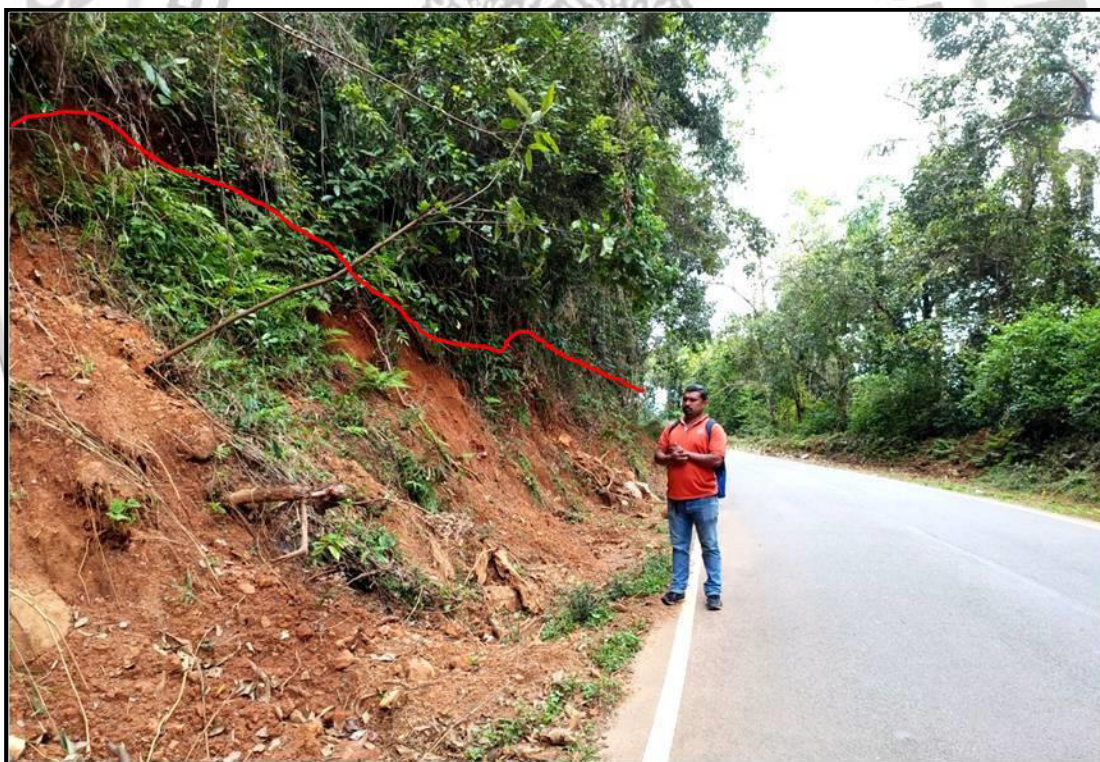
Fig. 5.12: A cut slope along Bhagamandla Talakaveri road near Cherengala
